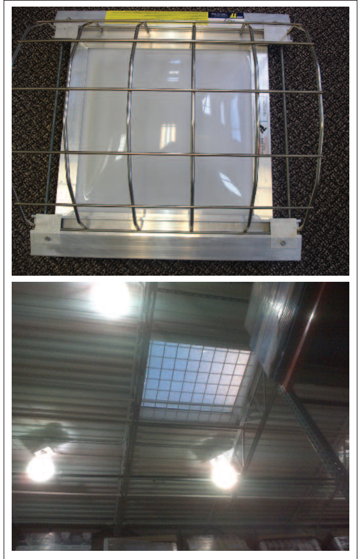
Exterior and interior skylight fall protection
