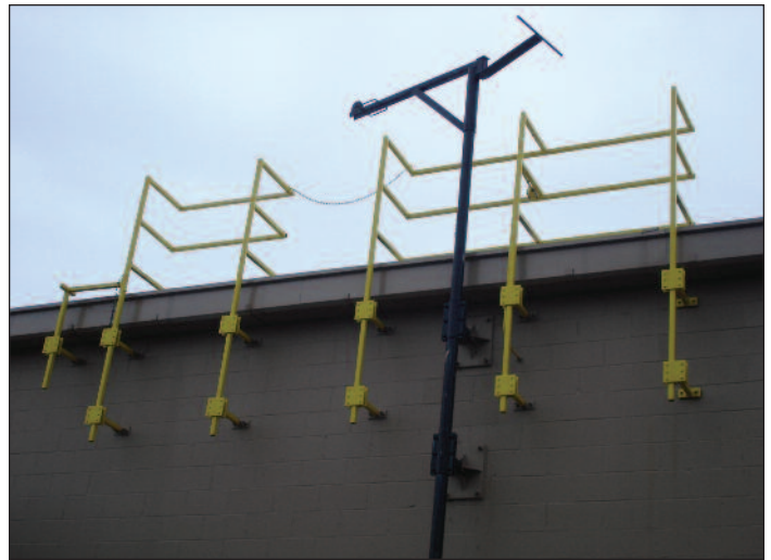
Integrated guardrails for permanent equipment hoist
