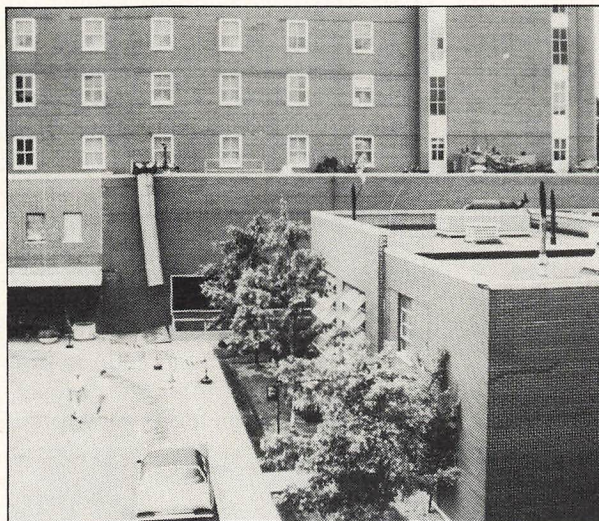
A tear-off chute and warning flags are set in place while Midland works on reroofing a section of Memorial Hospital.
