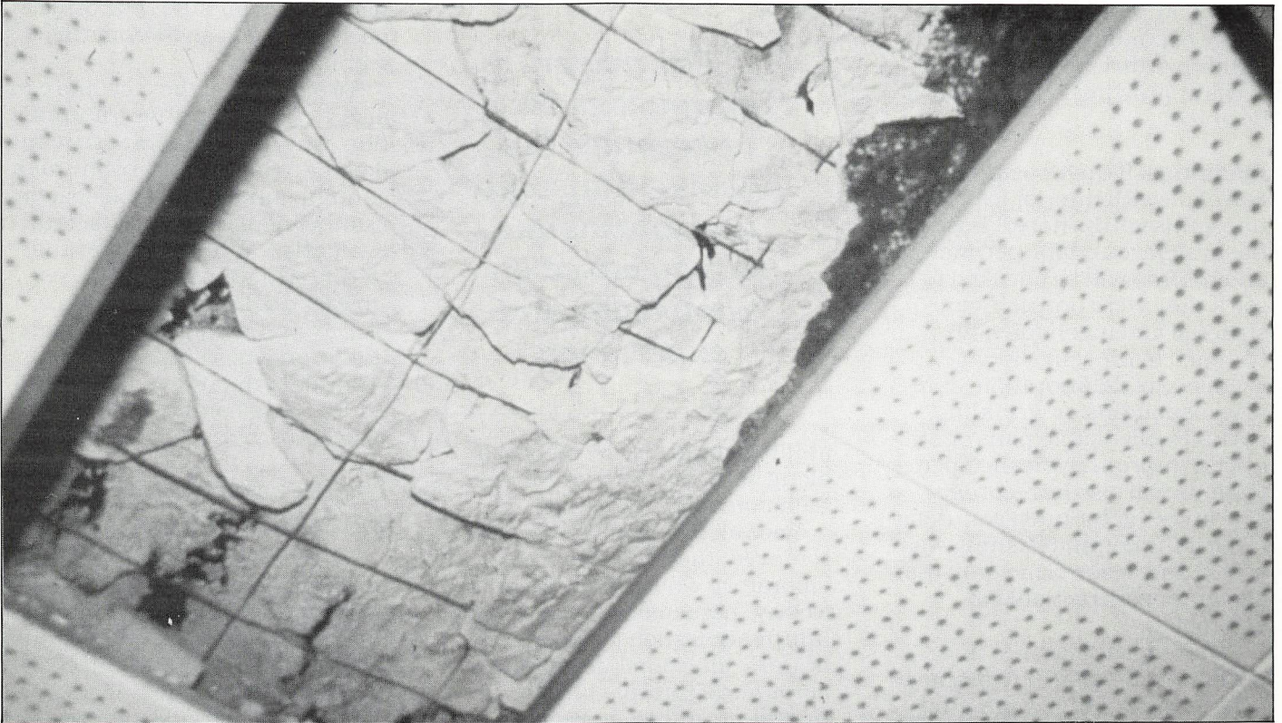
Examining the underside of the roof may be the only way to discover this type of deteriorated condition.
