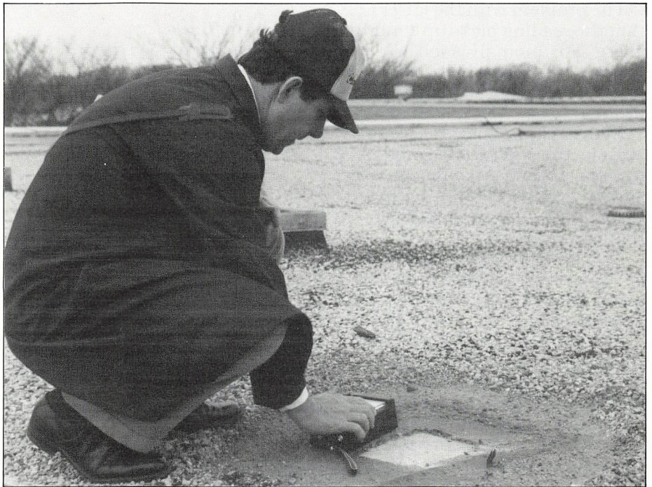
An investigator places a hand-held electrical capacitance meter on a roof surface to measure roof moisture.
