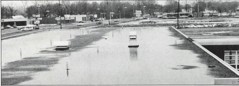
If large ponds such as this remain on the roof longer than 24 hours after a rain, it may indicate the need for reroofing to correct the condition.
