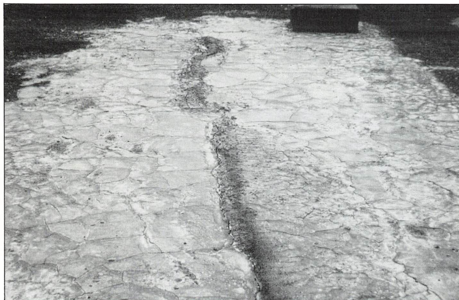
Roof problems such as ridging, alligatoring, cracking and blistering will be documented in the investigator's report.
