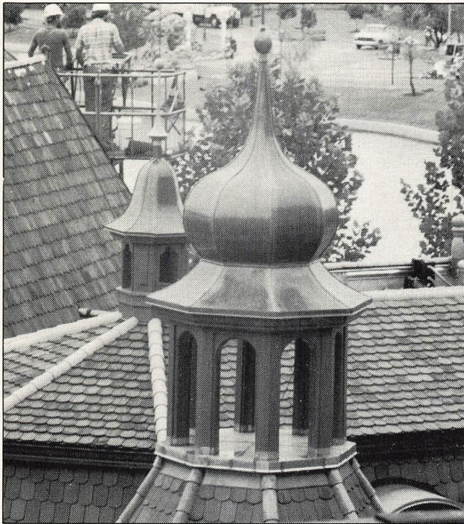
A terne-metal roof tower resembles its German counterpart under the direction of Giffen Roofing Co.
