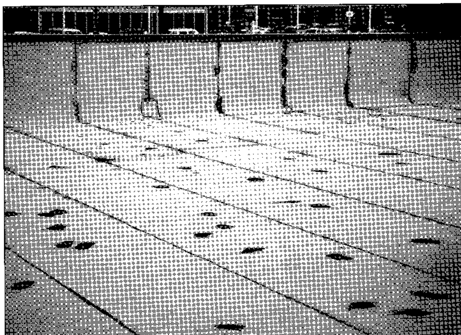
Photo 47. Roof 16: This granule-surfaced APP modified bitumen membrane (which was composed of a cap sheet and a base sheet over phenolic insulation) was punctured by hail in a number of locations. The dark spots are where emergency repairs were made with asphalt roof cement. This two-year-old roof is located in Kansas City.
