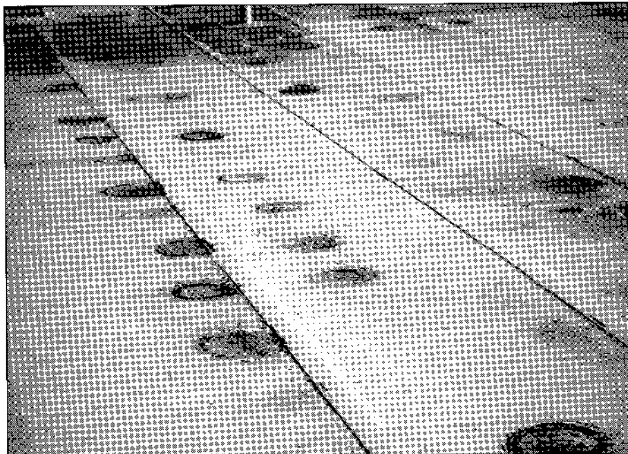
Photo 20. At another area of Roof 49, delaminations occurred above screw-and-plate fasteners that were used to attach the insulation, as depicted by the large diameter dark circles. A test cut at one of these areas revealed the separation occurred in the same location as described in Photo 19. Although in this case, the portion of the sheet above the separation was not deteriorated, as it was in Photo 19.
