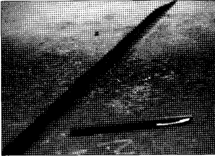
Photo 32. Roof 2: Lap separation (lifting and peeling) of a self-adhering polymeric-surfaced SEPS membrane roof is shown. This separation occurred in a ponded area. The age of this roof, which is located in Chicago, is unknown.
