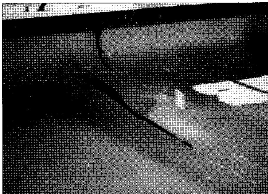
Photo 35. Roof 17B: The cap sheet lap has nearly pulled apart near the top of this large blister. This five-year-old SBS modified bitumen membrane is located in Kansas City. Although in many instances blister repair is not needed, this illustrates a condition where repair is important.
