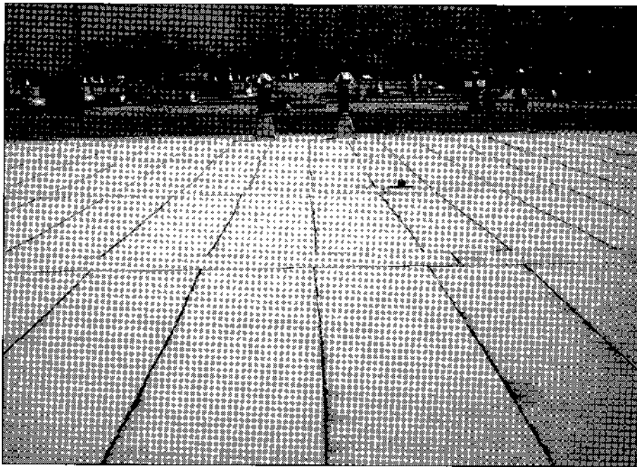
Photo 33. Roof 6: Several of the APP modified bitumen sheets on this roof exhibited hooking. This two-year-old roof is located in Chicago.
