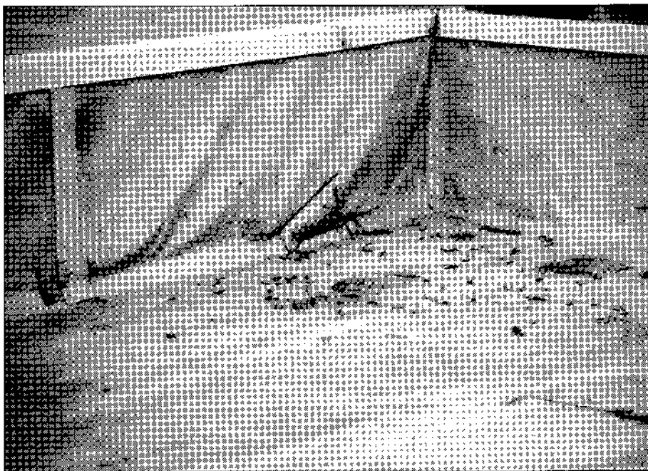
Photo 5. Roof 61: APP modified bitumen base flashing has separated from the parapet. The diagonal wrinkles are indicative of differential movement between the parapet and the roof deck. In several areas near the ink pen, the flashing is severely cracked. This five-year-old roof is located in New Orleans.
