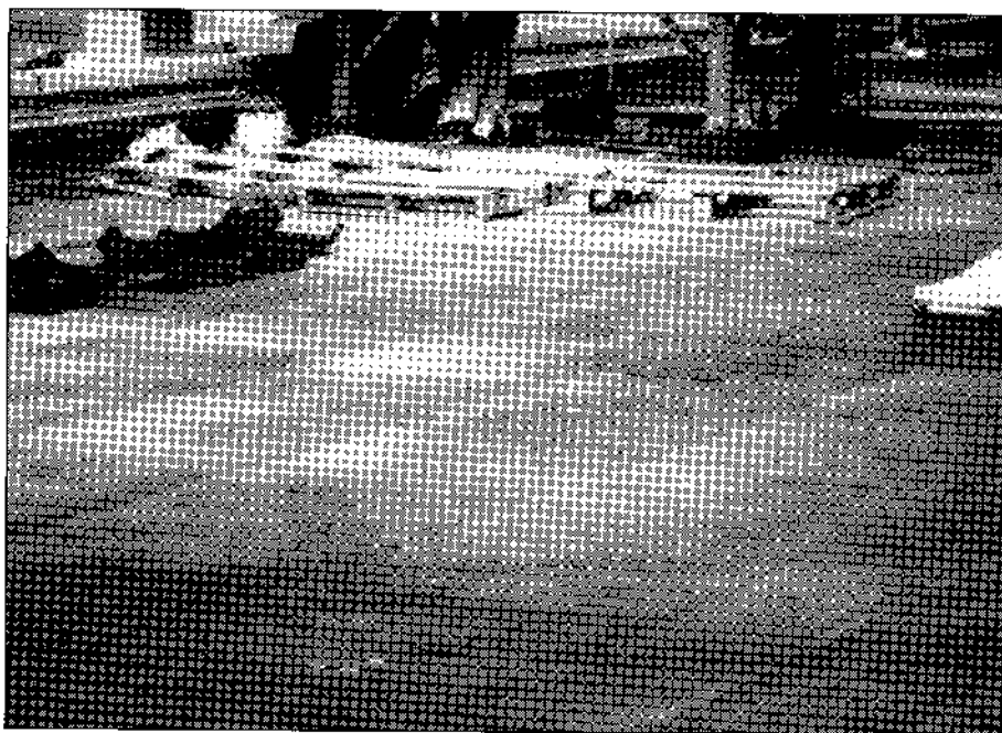
Photo 46. Roof 4A: Wood pallets and heavy pieces of steel and other material are laying on the membrane of this manufacturing facility. The membrane has been punctured in the foreground, near the ink pen. This nine-year-old APP modified bitumen membrane is located in Chicago.
